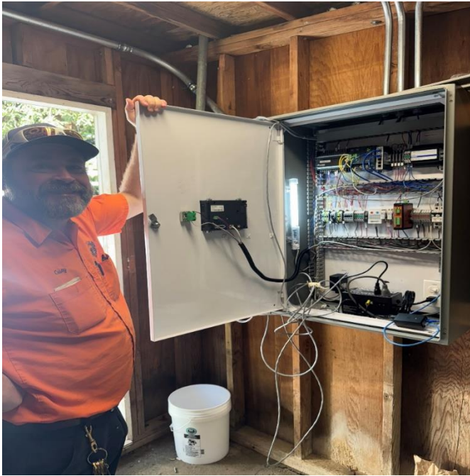
Labre SCADA panel 03/24/2025
